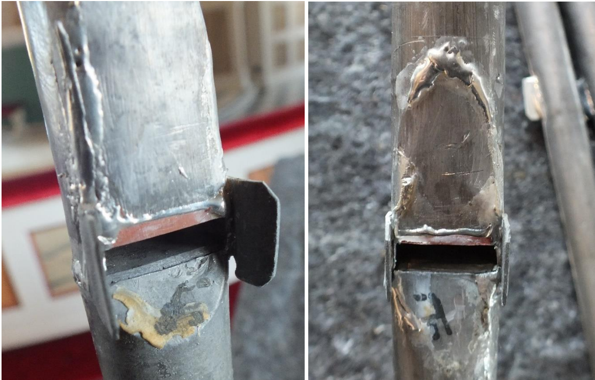
Photo 69, 70: non-professional treatment of the pipes
