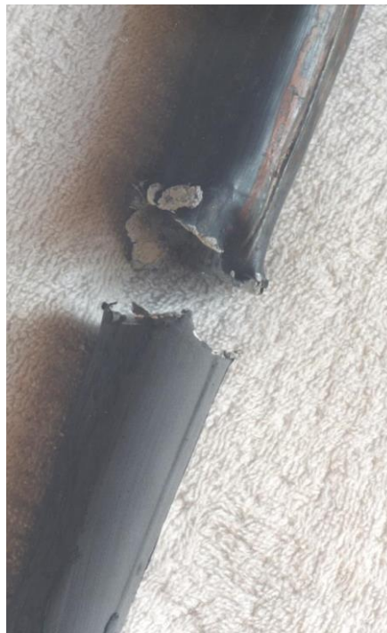
size (glue & white chalk) not being washed off the inside after soldering but accumulating moisture on the thin lead material
