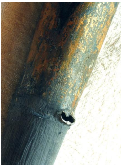
Damages on those 2 pipes as found in March 2000, just where new pipe foot tips were soldered on c. 1960. The new lower part disguised by paint. This calamity only stems from the pipemaker's
